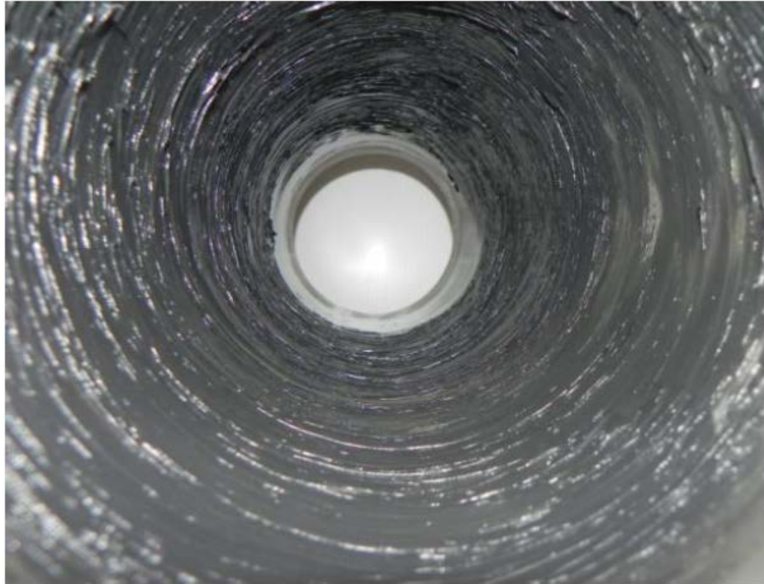
Fig.17. Meter body covered with black grease
